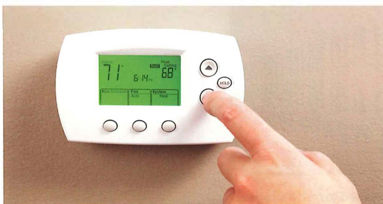
Figure 6.03 A thermostat can be used to control the temperature in a home or work place
